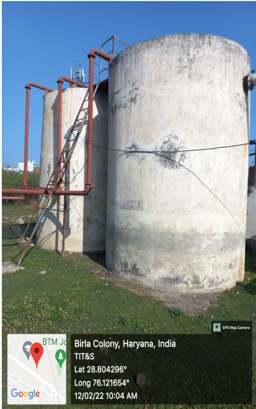
Waste water recycling (STP): view5
