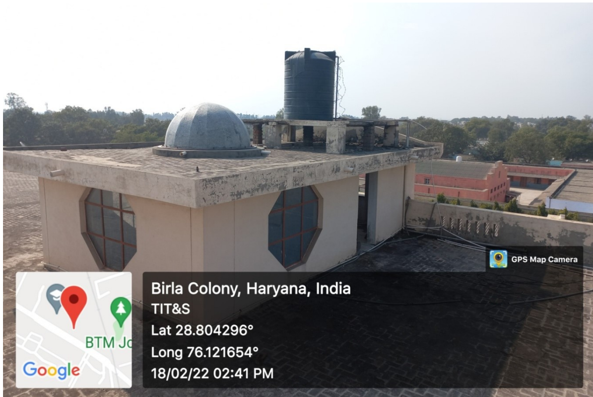
Water tank and distribution system
