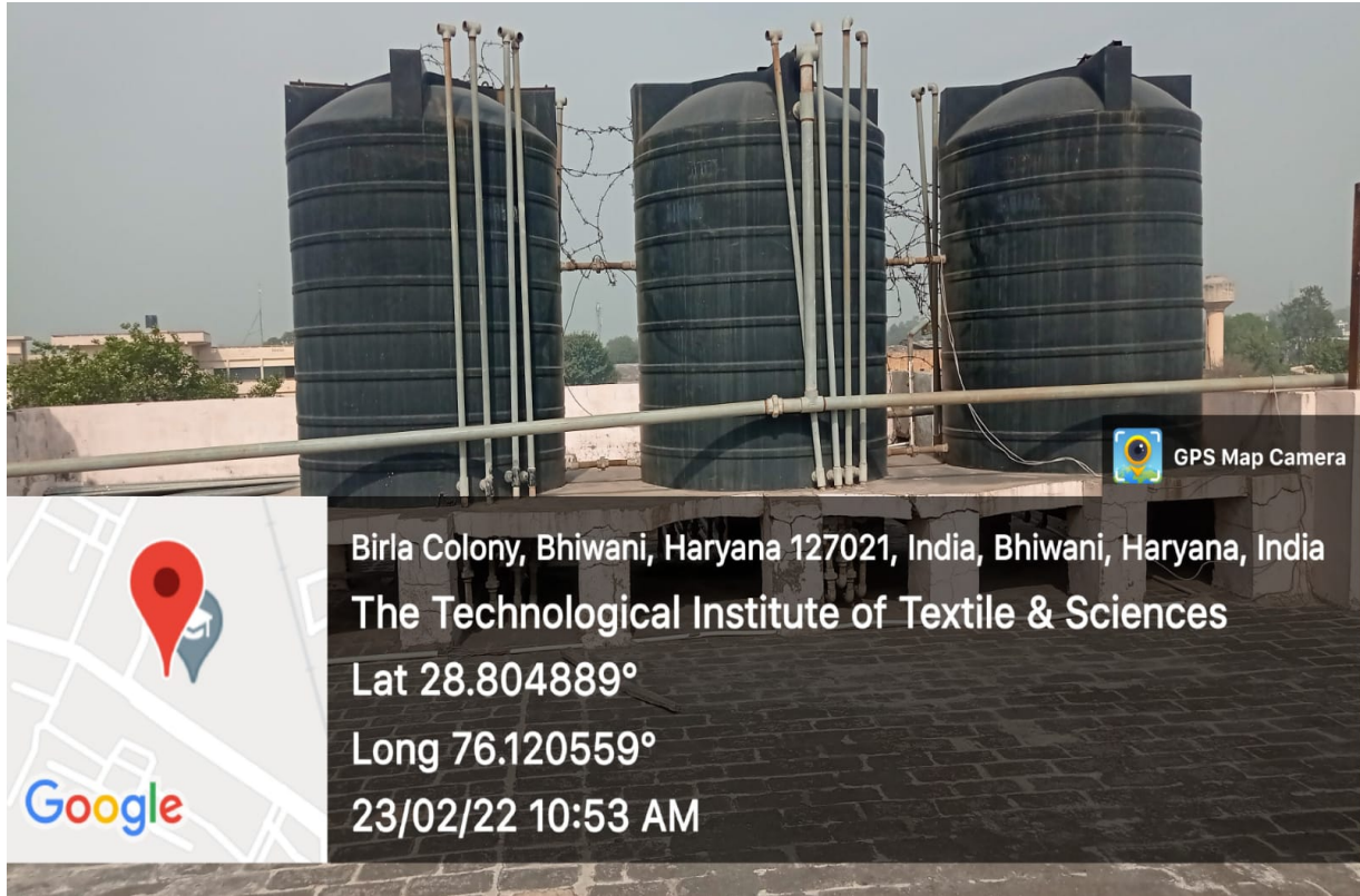
Water tank and distribution system
