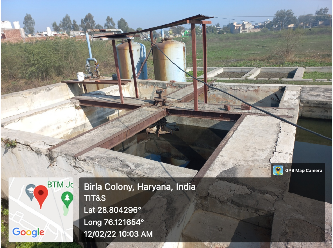
Waste water recycling (STP): view2
