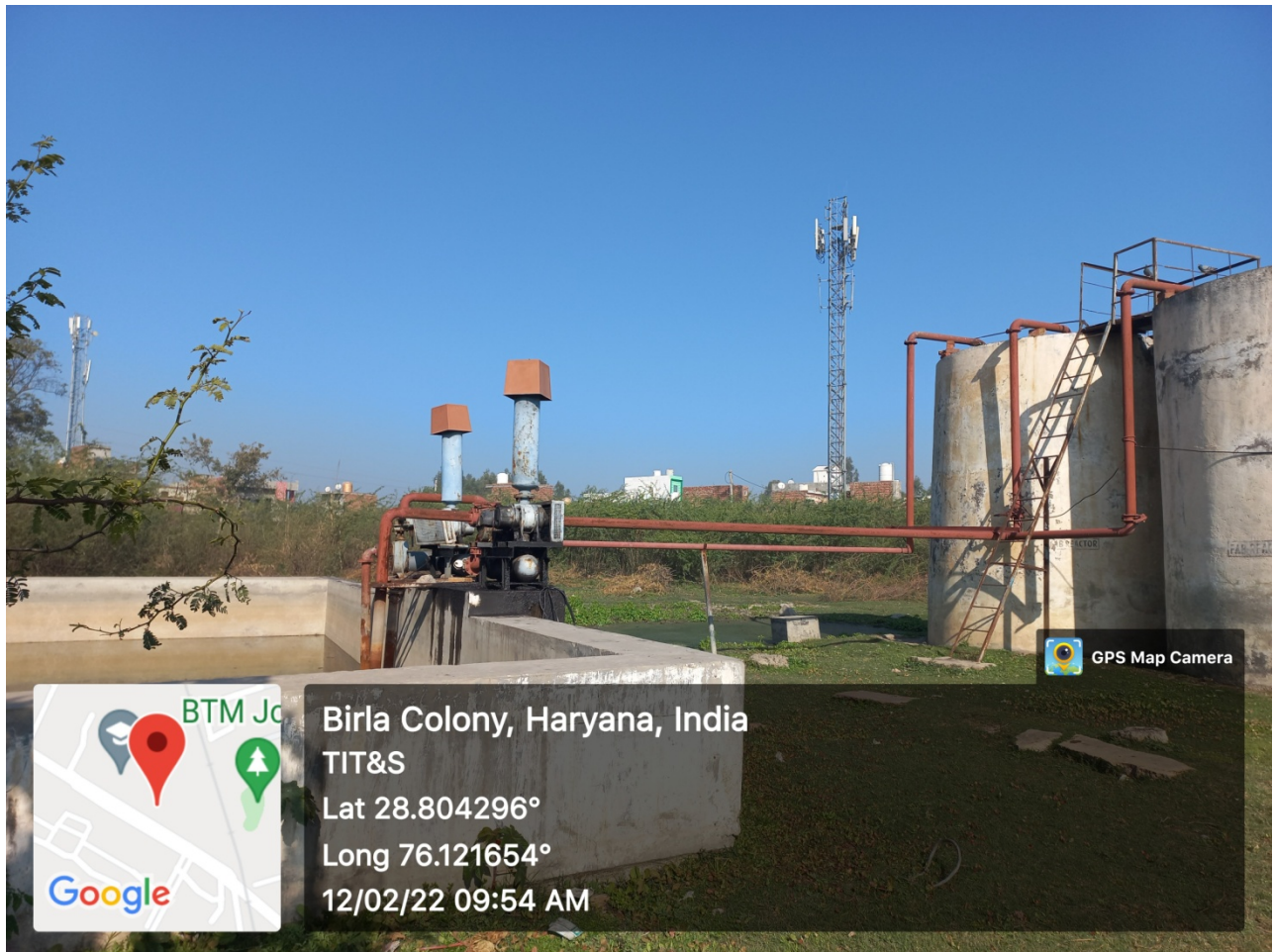
Waste water recycling (STP): view3
